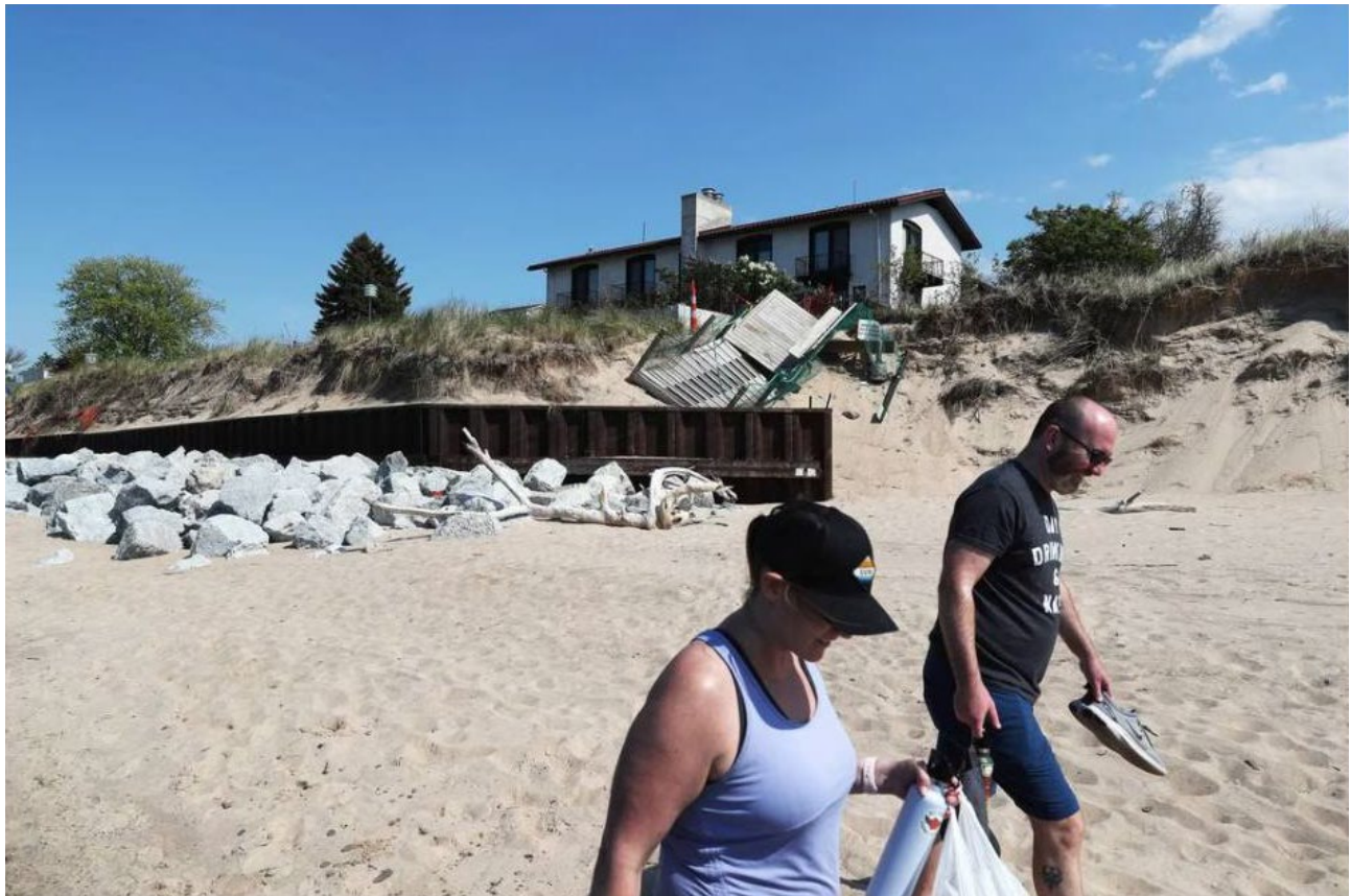
Beachgoers walk past boulders, an exposed retaining wall, and a damaged walking path on Ogden Dunes Beach at Ogden Dunes in Portage Township, Ind., on Friday, May 14, 2021. Erosion in recent years required the placement of boulders along the beach in 2020 to protect homes, but more beachfront has appeared in 2021. (John J. Kim/Chicago Tribune) (John J. Kim/ Chicago Tribune)
